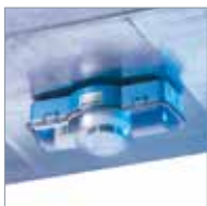
Smoke detector in duct
